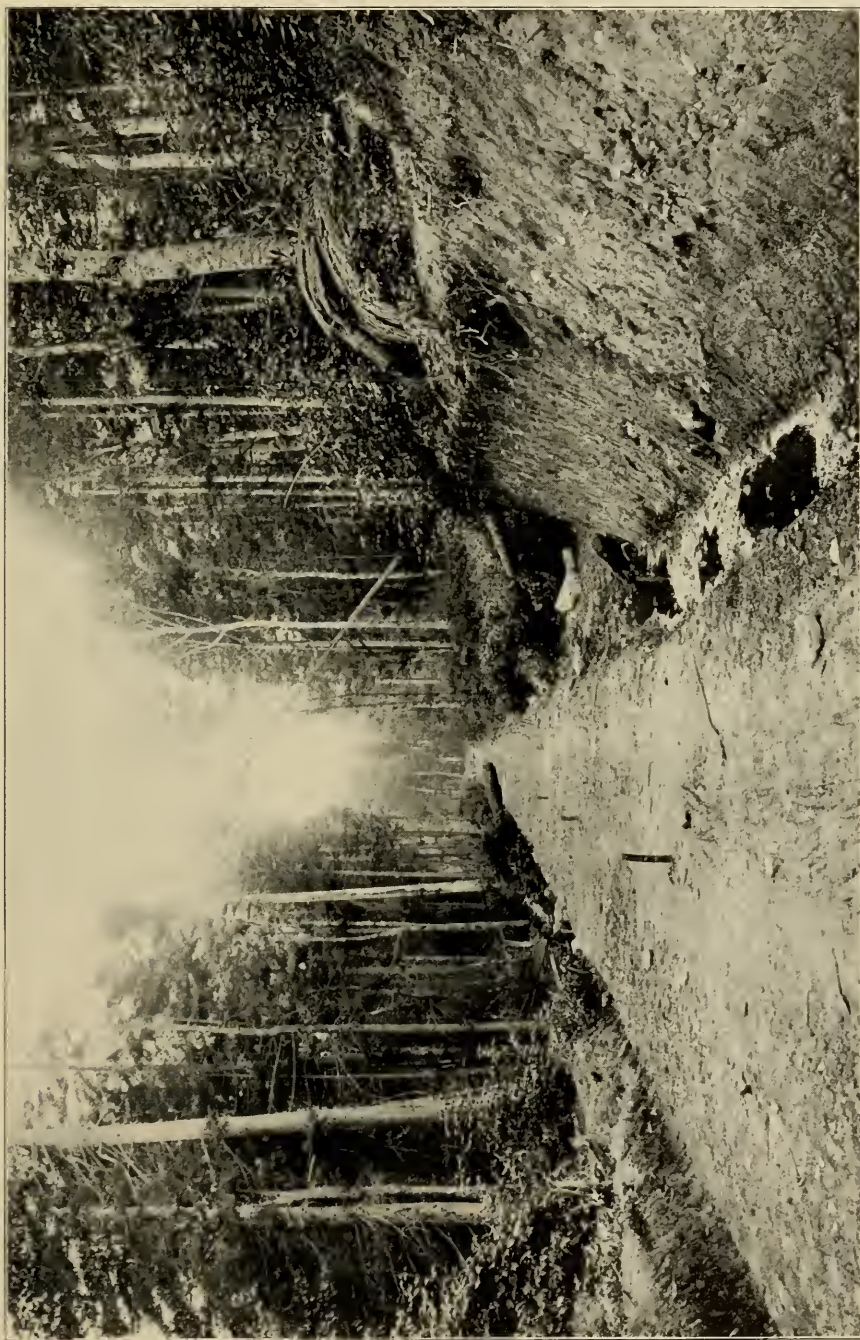
PLATE LXXI.—Grade for a lumber railroad near head of Cranberry River. (Photo, republished from page 68 of Volume V of the Survey).
